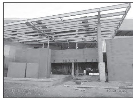
Construction on the River People Health Center project at McDowell Road and the Beeline Highway continues and will be utilizing various trades over the next year. Photos submitted by ECS
