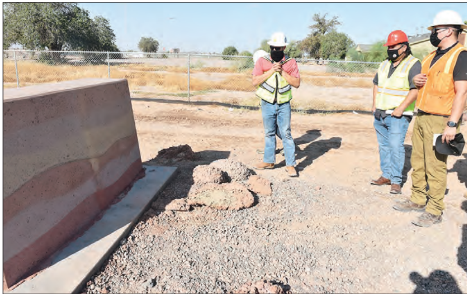
The Cultural Resources Department take a look at how the exterior walls will look like on the Repository and NAGPRA buildings.
