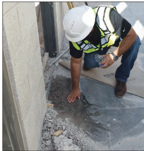
David Dallas, President of MayDall Construction shows guests who toured the new Repository how the interior flooring will look, the concrete flooring was grinded down to show the rocks inside; representing the river bottom.
