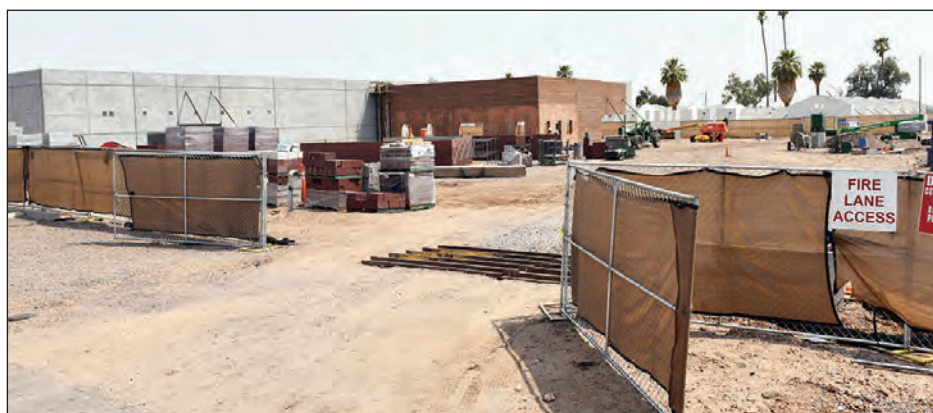
One of two Engineering and Construction Services (ECS) projects that have continued progress throughout the COVID-19 pandemic is the Cultural Resources Department's new Repository building. Crews have continued construction and made great progress.
