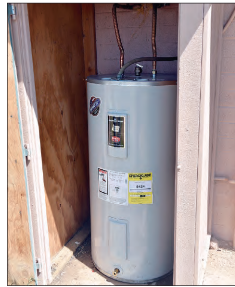
Water heater replacement is just one of the many services that SHRRP provides for SRPMIC senior and disabled members.
