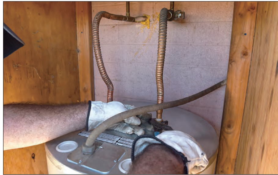
SHRRP Plumber Dave Black starts his day off replacing a water heater for a SHRRP customer, he makes sure everything is tightened and ready for use.
