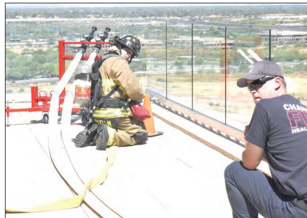
Fire staff connect hoses and prepare for the water pressure tests to be conducted.
