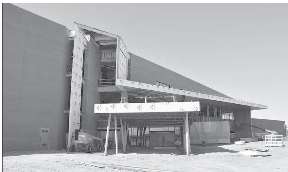
River People Health Center. The yet-unnamed dental suite will be housed on the second floor.
