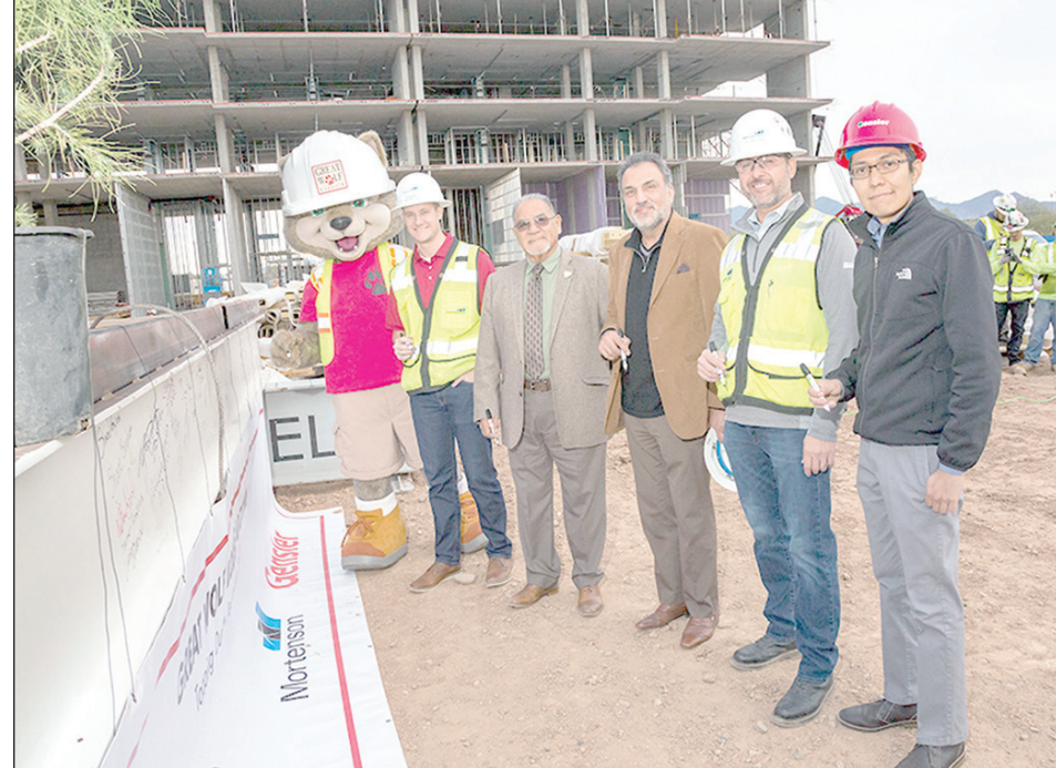
One of the larger construction projects in the Talking Stick Entertainment District celebrated another milestone with its "topping out" ceremony. Great Wolf Lodge Arizona has taken form near Salt River Fields in the northwestern part of the Salt River Pima-Maricopa Indian Community. On December 11, the destination family indoor water park resort hoisted into place the final steel beam of the structure. SRPMIC President Delbert W. Ray Sr. took part in the ceremony. Great Wolf Lodge Arizona is scheduled to open in late summer/early fall 2019. For details about the resort, visit www.greatwolf.com . Dalton Walker, O'dham Action News. (Photo courtesy of Great Wolf Lodge Arizona)
