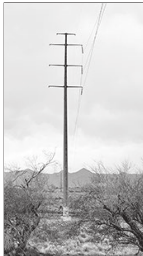
An example of a WAPA pole similar to the existing pole in the river. Photo courtesy of Tina Sotero
