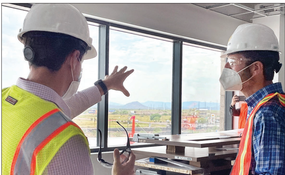
Engineering and Construction Services Senior Construction Manager Joshua Sciacca shows Stanton the view from the River People Health Care as they tour the entire building.
