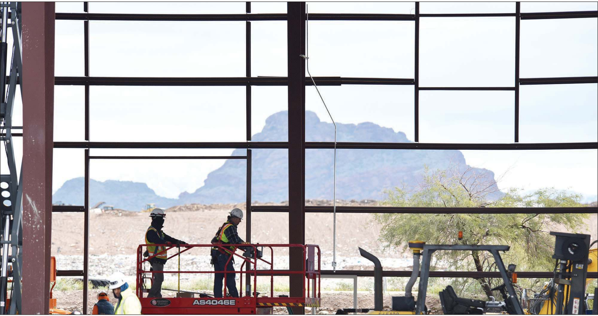
Workers constructing the new recycling facility at the Salt River Landfill, with Red Mountain and the rest of the landfill in the background.
