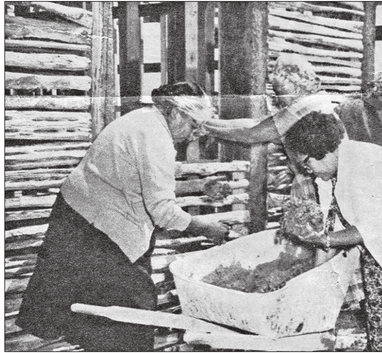
Community women help reinforce the building that is framed with saguaro ribs. Photos courtesy of the Huhugam Ki: Museum
