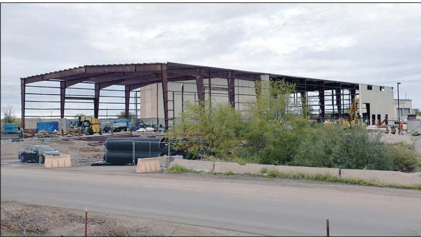
The new recycling facility at the Salt River Landfill being built and operated by Republic Services.
