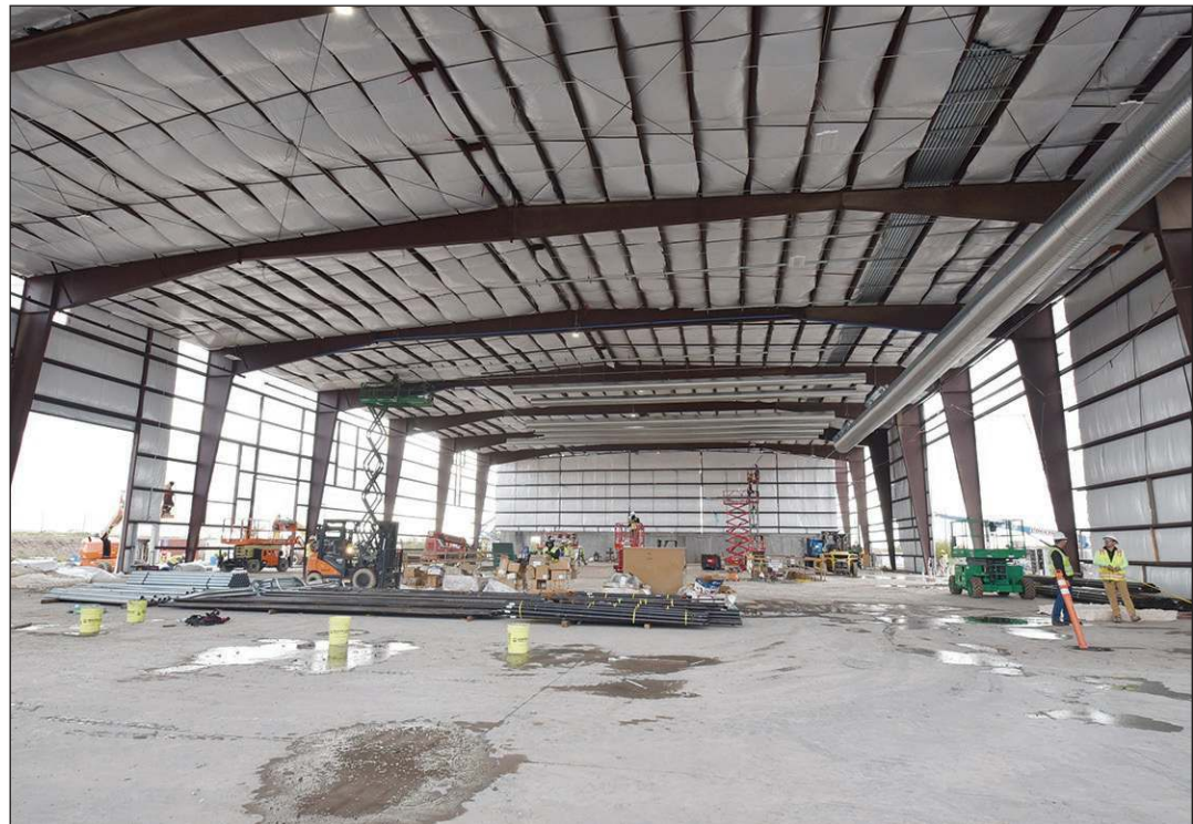
A wide look into the inside of the new landfill facility, with workers assembling parts of the building.
