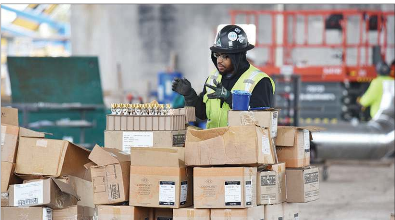
A worker going through parts that will end up in the construction of the new recycling facility.
