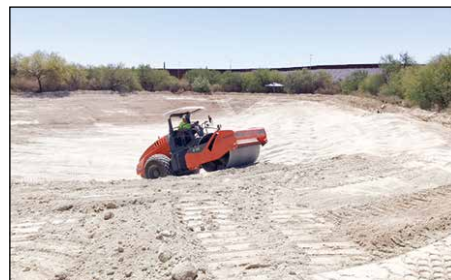
Construction crew continues replacing the old lining of Quitobaquito Pond. Photo courtesy of the National Park Service
