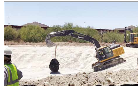
Construction crew works on replacing the lining of Quitobaquito Pond. Photo courtesy of the National Park Service
